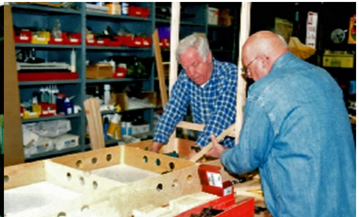
Dave Connery, on the left, and Ron Kolo working on the framing.
