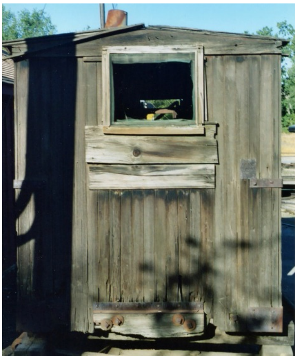
This view of the end of the car shows the buffer block well.
