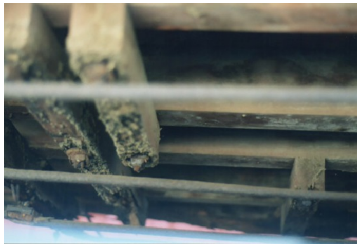
This view under the car between the needle beams shows what appear to have been mounting blocks for a brake system.
