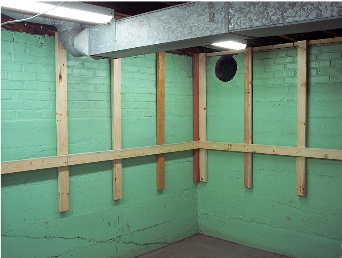
My brainstorm of attaching the 2 x 4’s to the sill to support the back of the layout.
