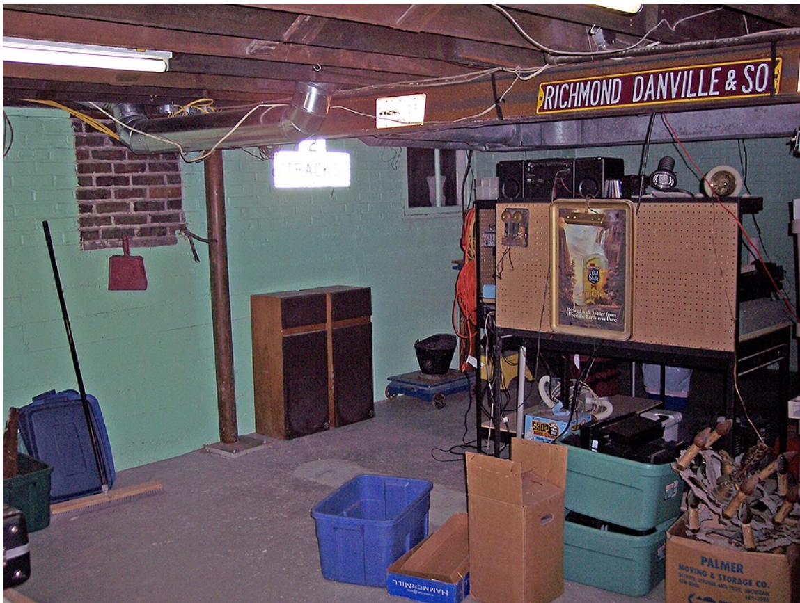
The wall gone and beam in place. Of course, we were told that house would again settle so don't do any plaster repairs for a few years. (Like I was going to worry about that.) You can see the actual color of the brick where the old fuse box was.
