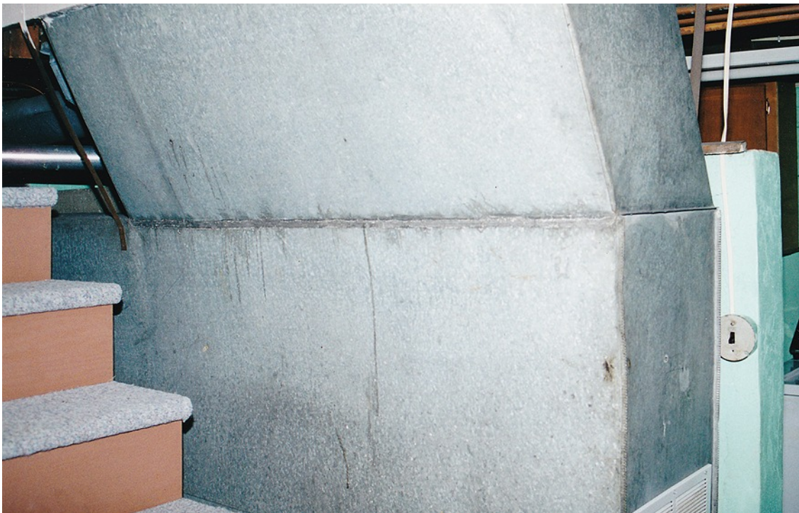
The single large cold air return was an eyesore and took up a lot of usable space. A new flexible pipe was installed. Still ugly, but much less space wasted. The half wall behind was the old cistern from back in the day, but does a nice job of blocking the washer and dryer, paint booth and toilet from the rest of the basement.
