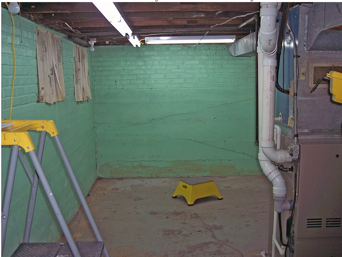
Cleaned up and installing the lighting. You can see where the poured concrete meets the brick. It's this area that drops down three inches.
