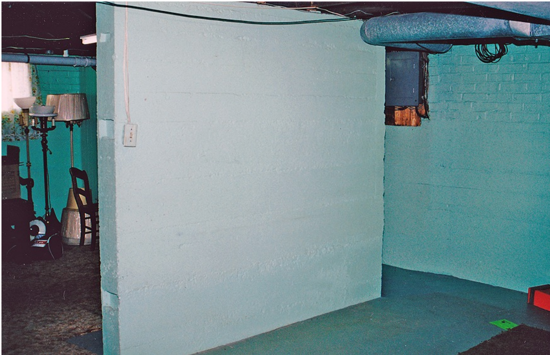
The wall that cut the basement in half and held the other three stories had to go. Note the beautiful green walls, shag carpet and the old fuse box – the joys of an old house.
