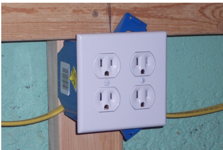
Outlets, you can not have too many of these. They are on a separate circuit from everything else.
