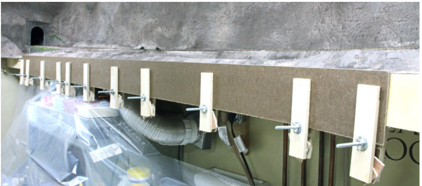
The final Masonite is being glued to the laminated fascia. Here, I flipped the clamps because of the height of the Masonite.
